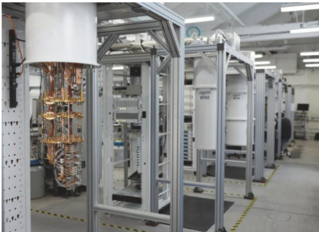
Rigetti's quantum computing facility in Berkeley, California includes both research and development and production quantum processing units, which are each housed in a dilution refrigerator.
