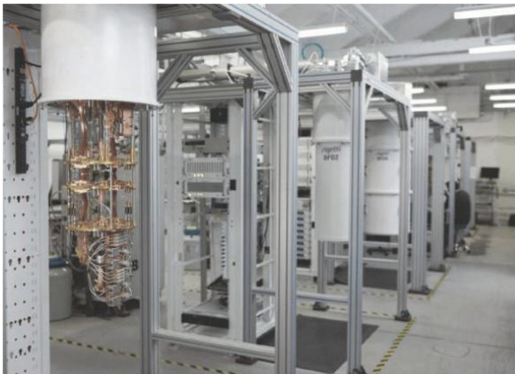
Rigetti's quantum computing facility in Berkeley, California includes both research and development and production quantum processing units, which are each housed in a cryogenic refrigerator.
