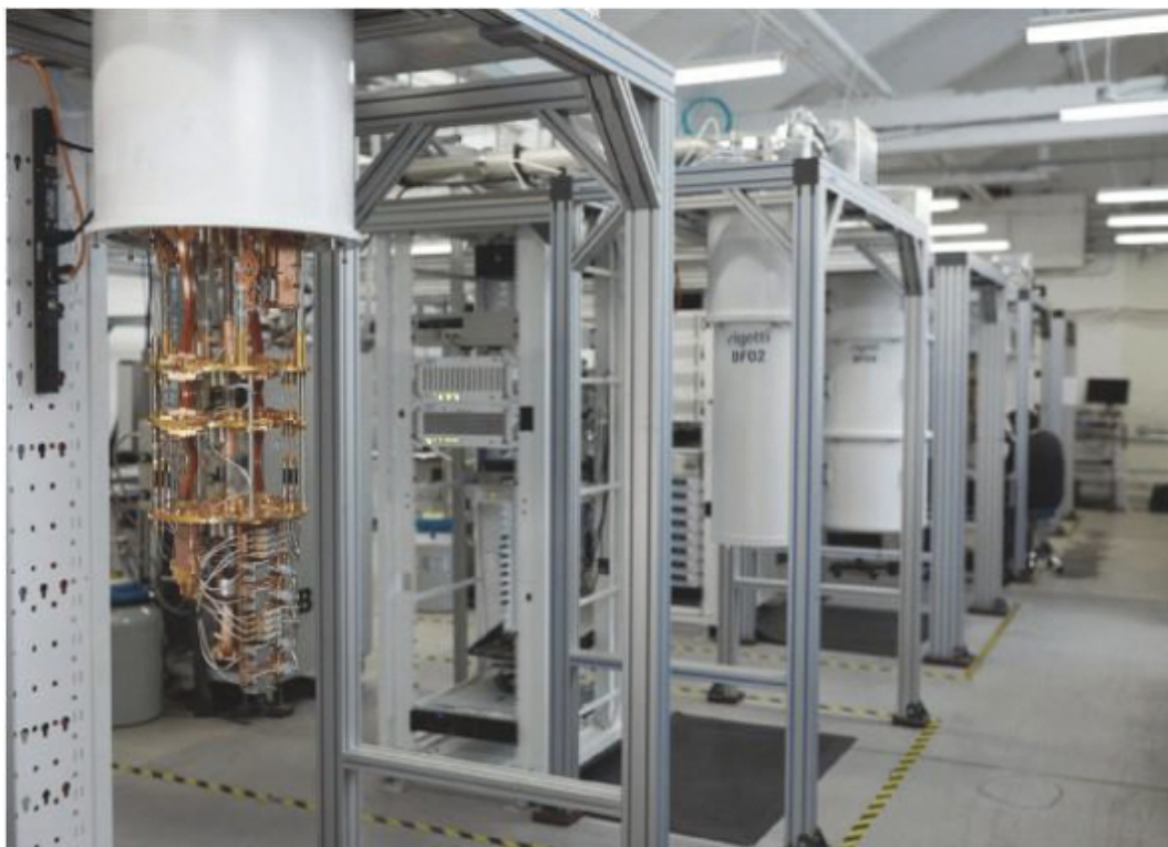
Rigetti's quantum computing facility in Berkeley, California includes both research and development and production quantum processing units, which are each housed in a dilution refrigerator.
